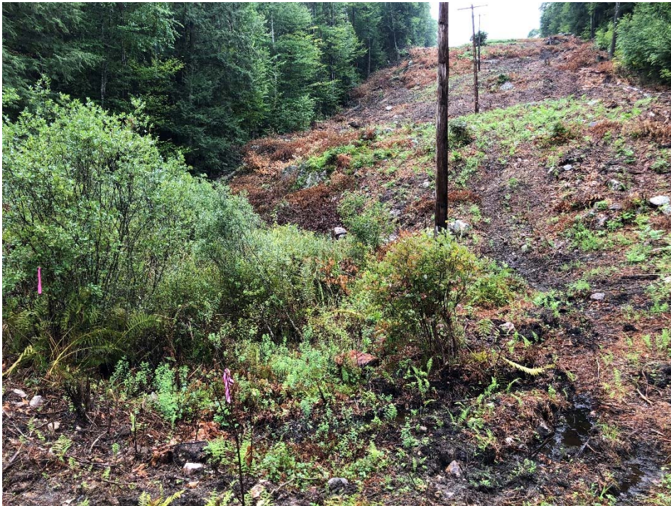
Photograph No. 4: Looking southwesterly at Wetland KW-1 and W110 Structure 2/179 to be replaced.
