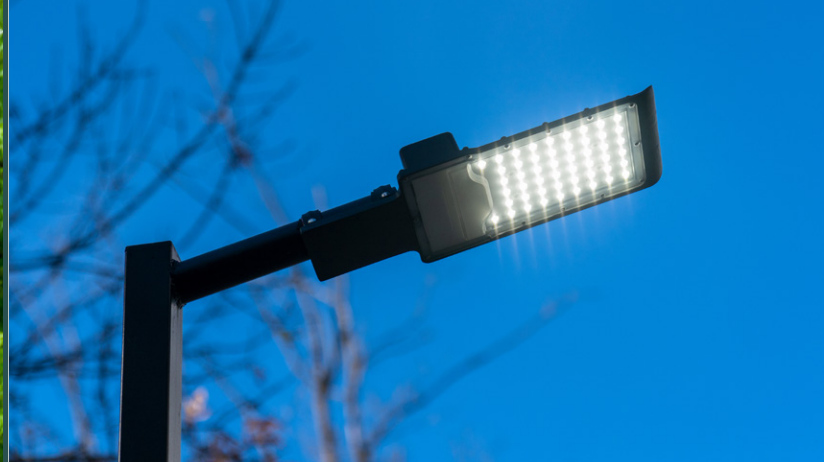
LED street lighting to enhance nighttime visibility for pedestrians and motorists.
