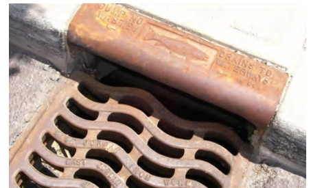
Marlboro Street Stormwater Drain to Beaver Brook
