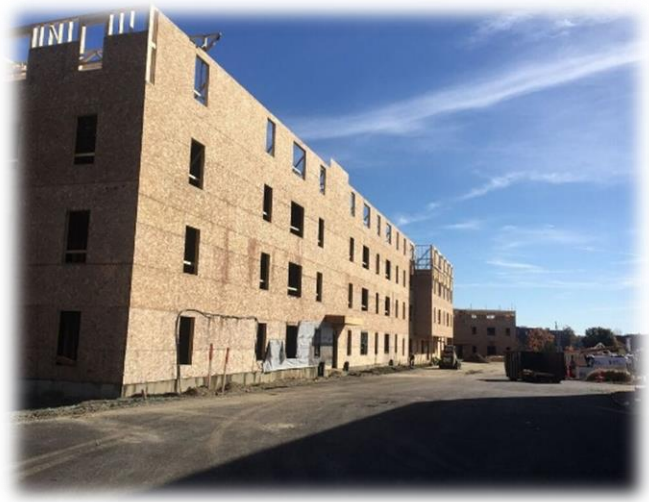
Figure 4.5. Construction of new apartments at Washington Park of Keene LLC. Source: Authors
