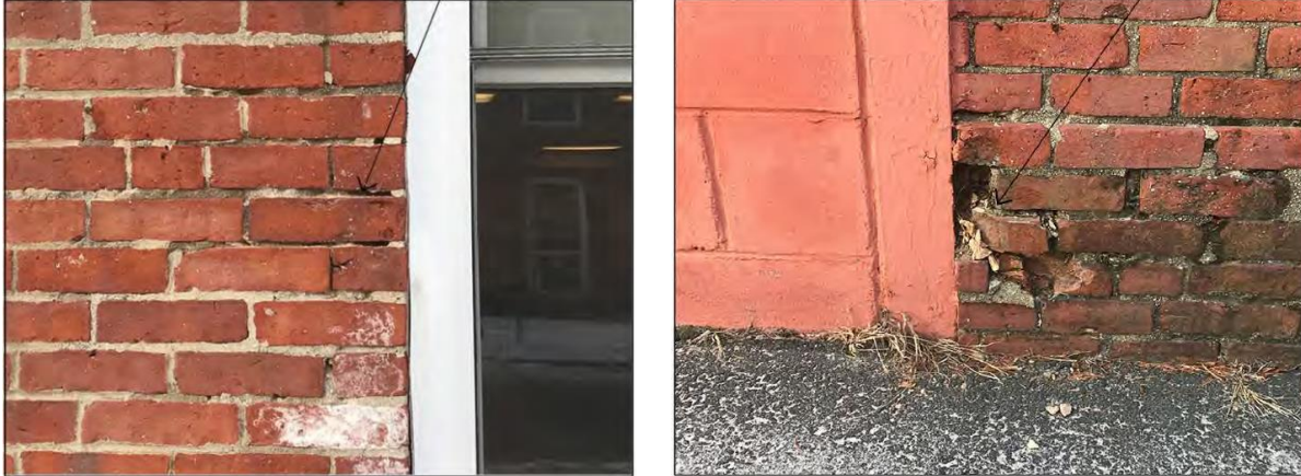
Above: Photographs of deteriorated mortar joints (left) and broken/damaged brick masonry (right) provided by applicant.
