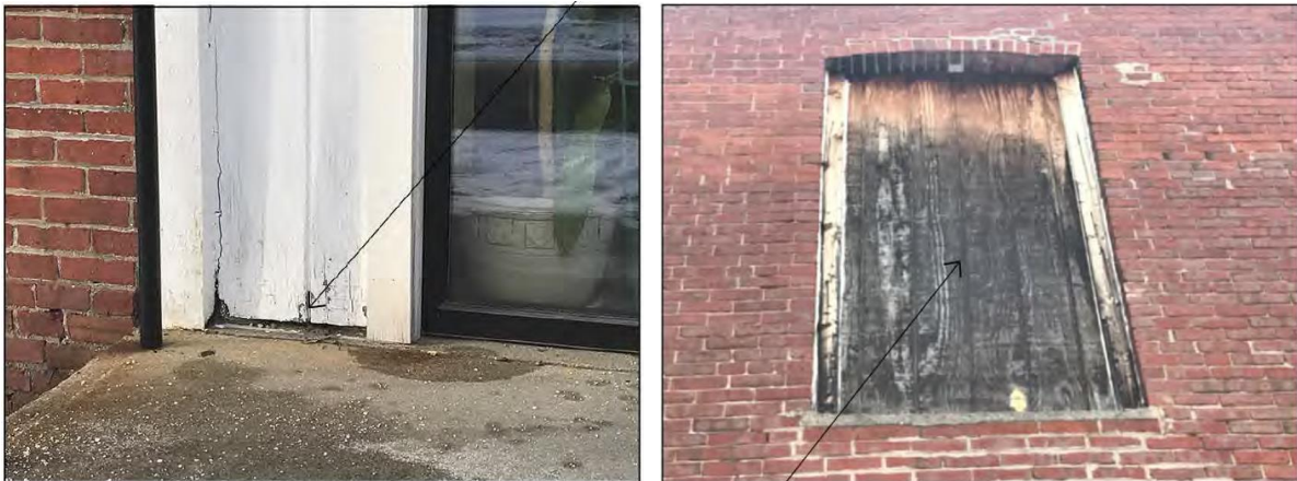
Above: Photographs of rotted wood trim on the front façade of the building (left) and existing window infill panels on the west side of the building (right) provided by applicant.
