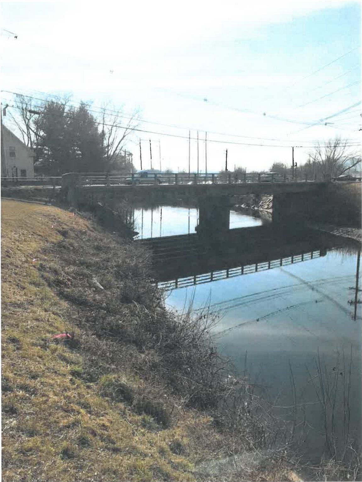
Photo 3: Winchester Street Bridge over the Ashuelot River facing downstream (Photo Direction: south)
