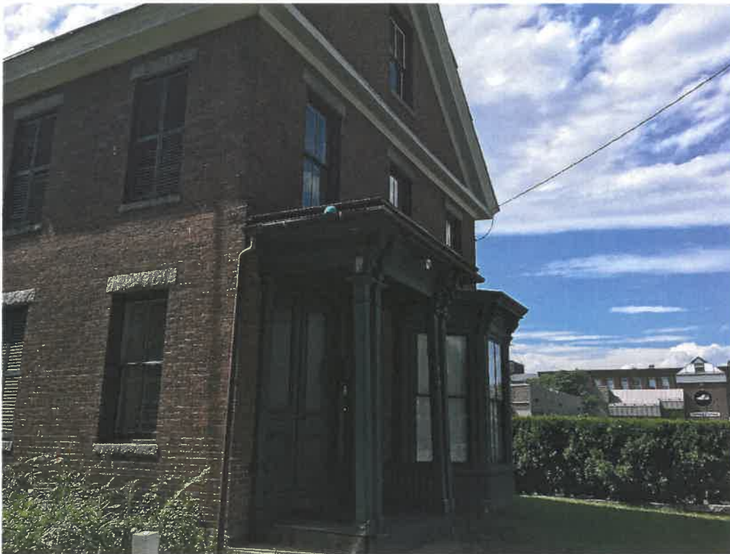
Image of front entry showing woodwork to be repaired and repainted and stairs to be reconstructed
