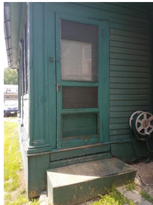
Left: View of door on south side of building proposed for replacement (outlined in red).
