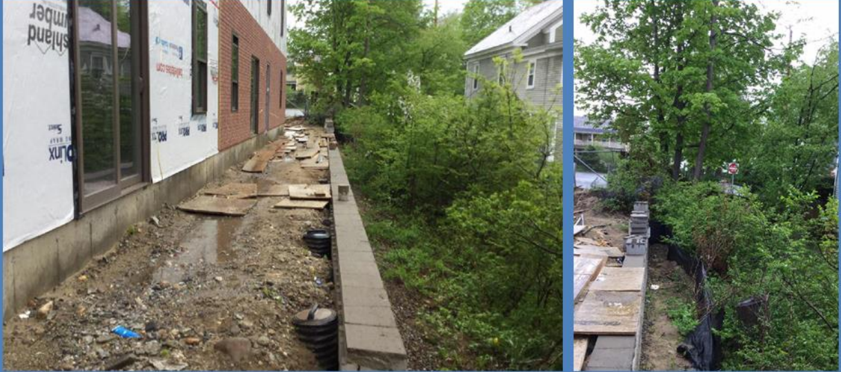
Northeast corner of property adjacent to 47 Spring Street in May 2018, with a 4' retaining wall & ~3:1 vegetated slope
