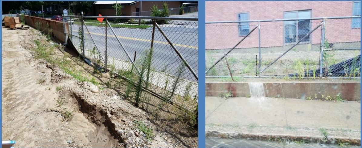
Runoff and sedimentation/erosion issues on Roxbury St. Photos taken 8/1/18
