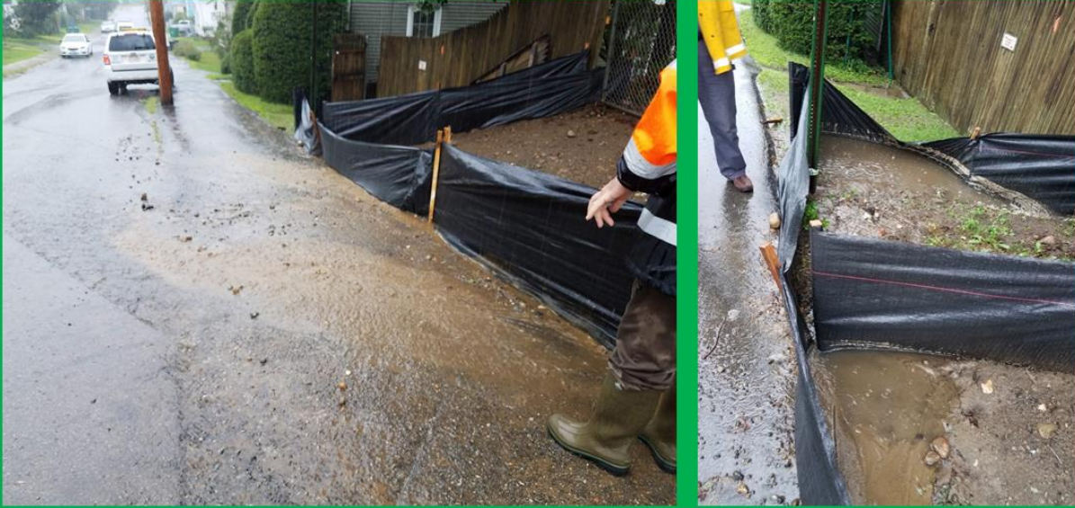
Runoff and sedimentation/erosion issues on Spring St. Photos taken 8/1/18
