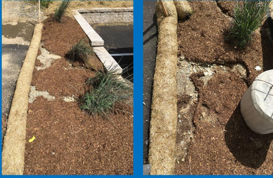
Runoff and sedimentation/erosion issues along site boundary with MoCo Arts property, behind the former Middle School building
