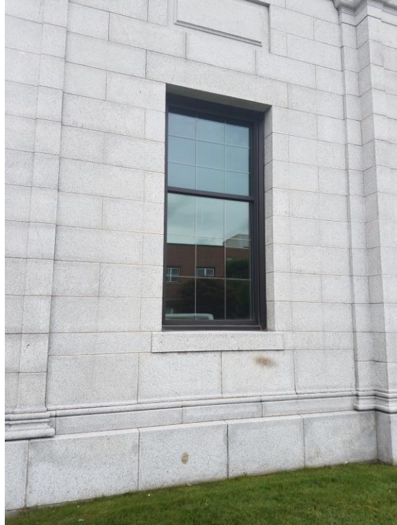
FIGURE 2: Photograph of replacement window taken on 9/10/18.
