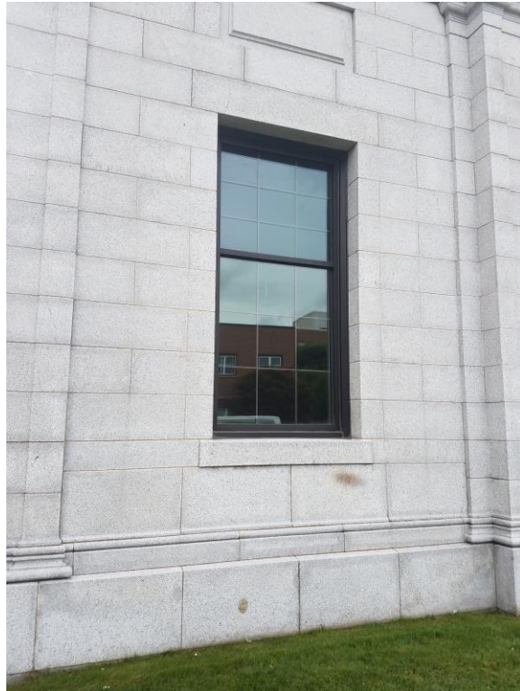
FIGURE 2: Photograph of replacement window taken on 9/10/18.
