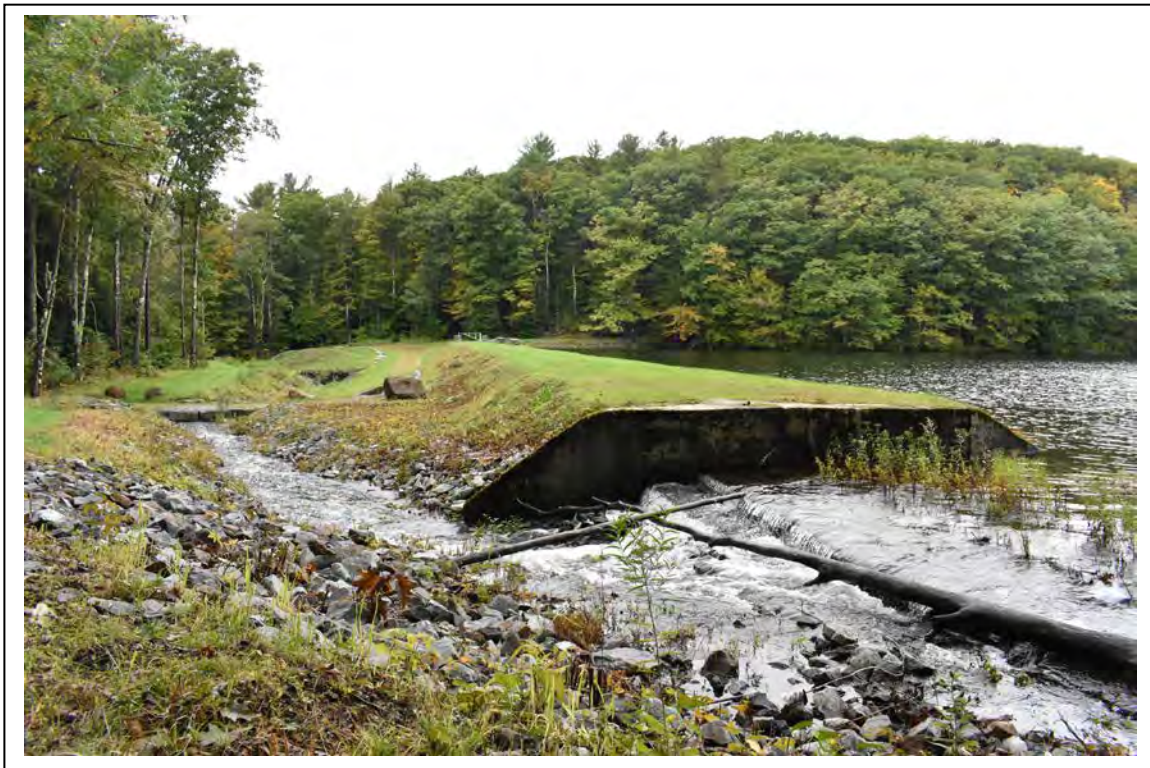
Photo # 3 Description: General view of sluiceway, sluiceway west abutment, and dam from east abutment. Reference (file name or frame#): ROX0006-03 Direction: West
