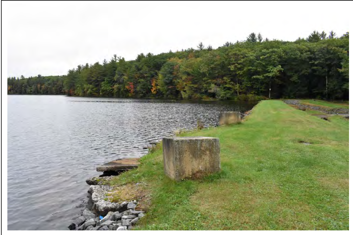
Photo # 2 Description: General view of dam, impoundment, and sluice intake area from dam crest. Reference (file name or frame#): ROX0006-02 Direction: Northeast
