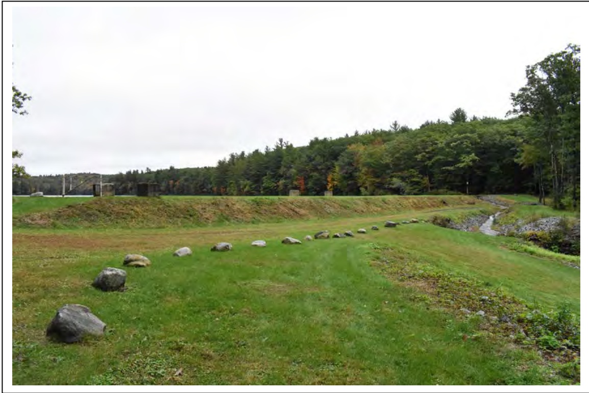
Photo # 4 Description: General view of downstream face of dam and spillway from 2010 terracing. Reference (file name or frame#): ROX0006-04 Direction: Northeast
