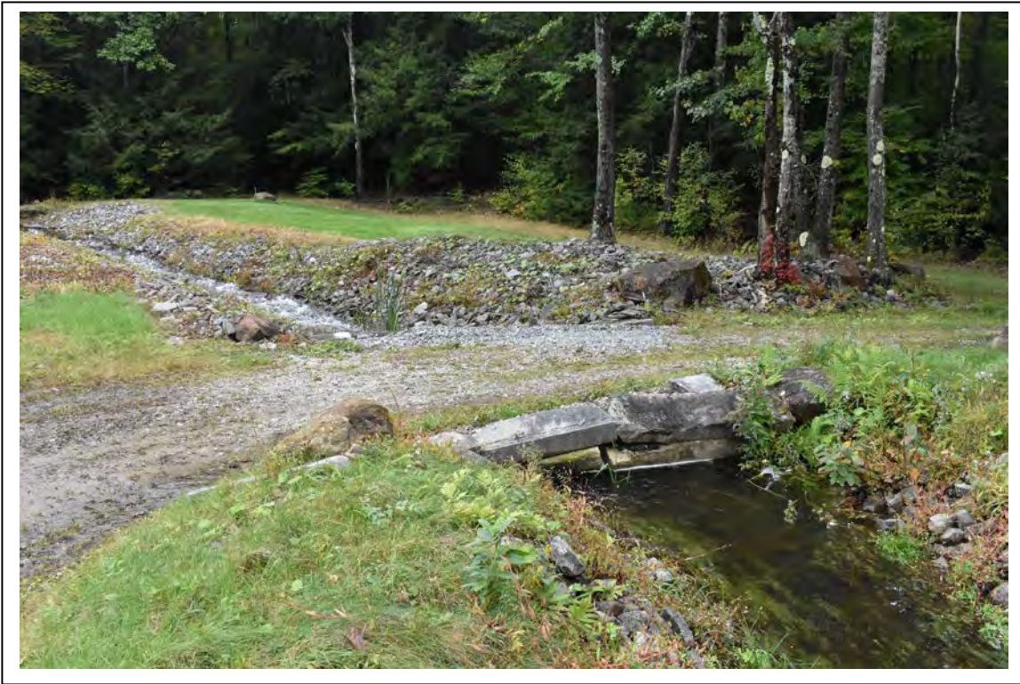
Photo # 8 Description: View of spillway channel and cut granite culvert from Woodward Pond Road. Reference (file name or frame#): ROX0006-08 Direction: East
