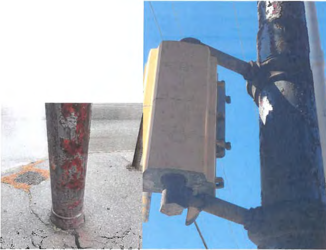
One of two main signal support poles. Hollow steel, both are ancient and badly corroded. One is missing its protective top cap, resulting in exposure to rain, snow and wildlife Typical fixture attached to steel pole. Severe corrosion all around, including the near amputation of the fixture's bottom connector
