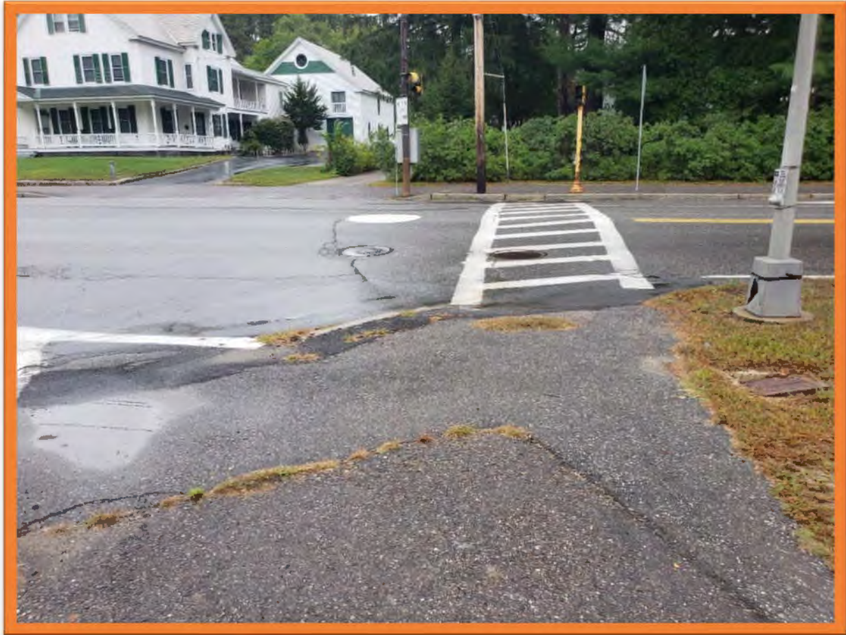
Example of non-ADA compliant ramps across Park Ave.
