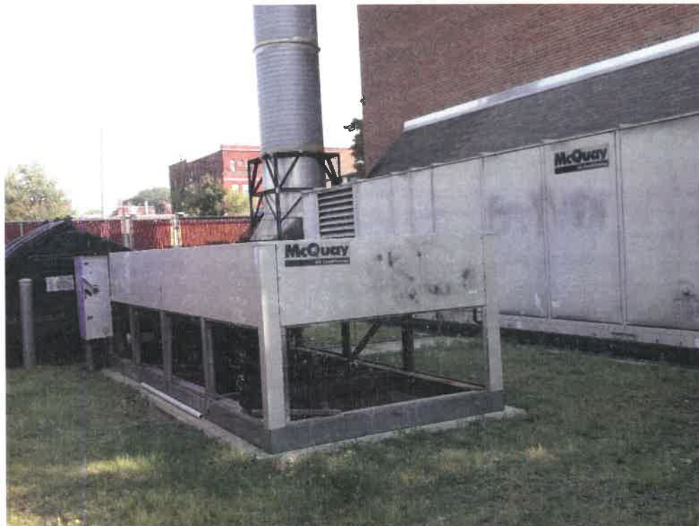
Figure 7 - existing HVAC equipment
