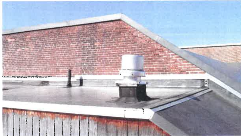
Figure 6 - example of brickwork requiring repointing
