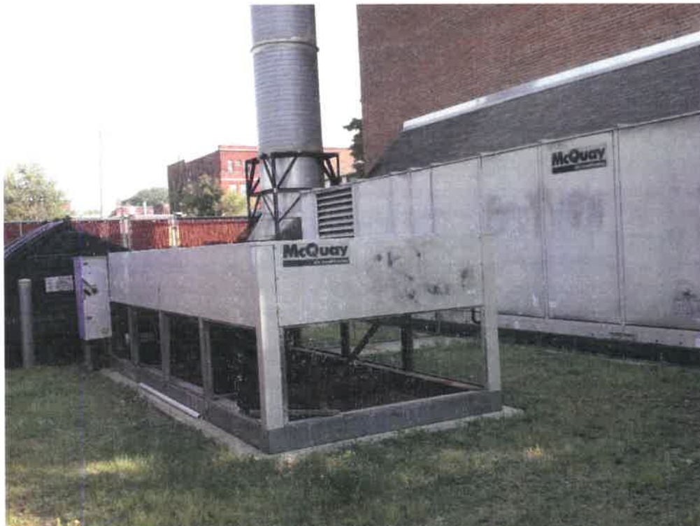
Figure 7 - existing HVAC equipment
