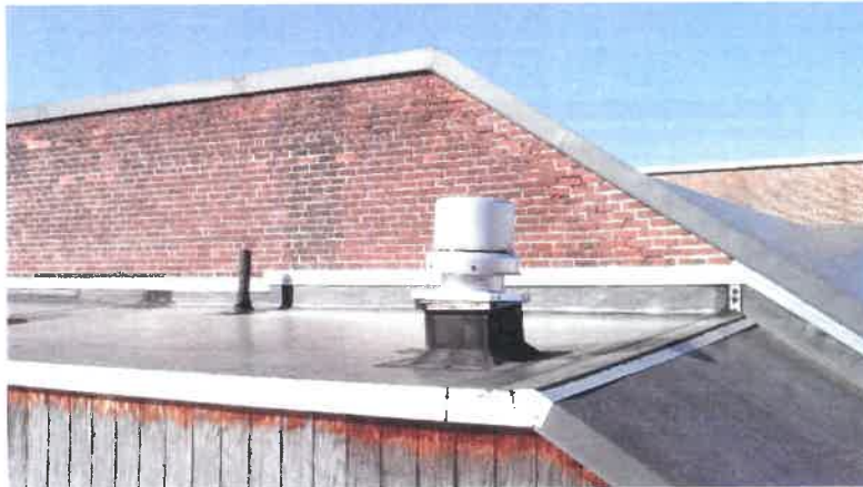
Figure 6 - example of brickwork requiring repointing
