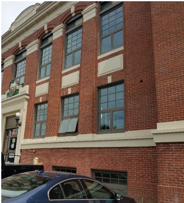
Figure 1. Image of 4-inch diameter penetration on the west façade of the former Middle School building.
