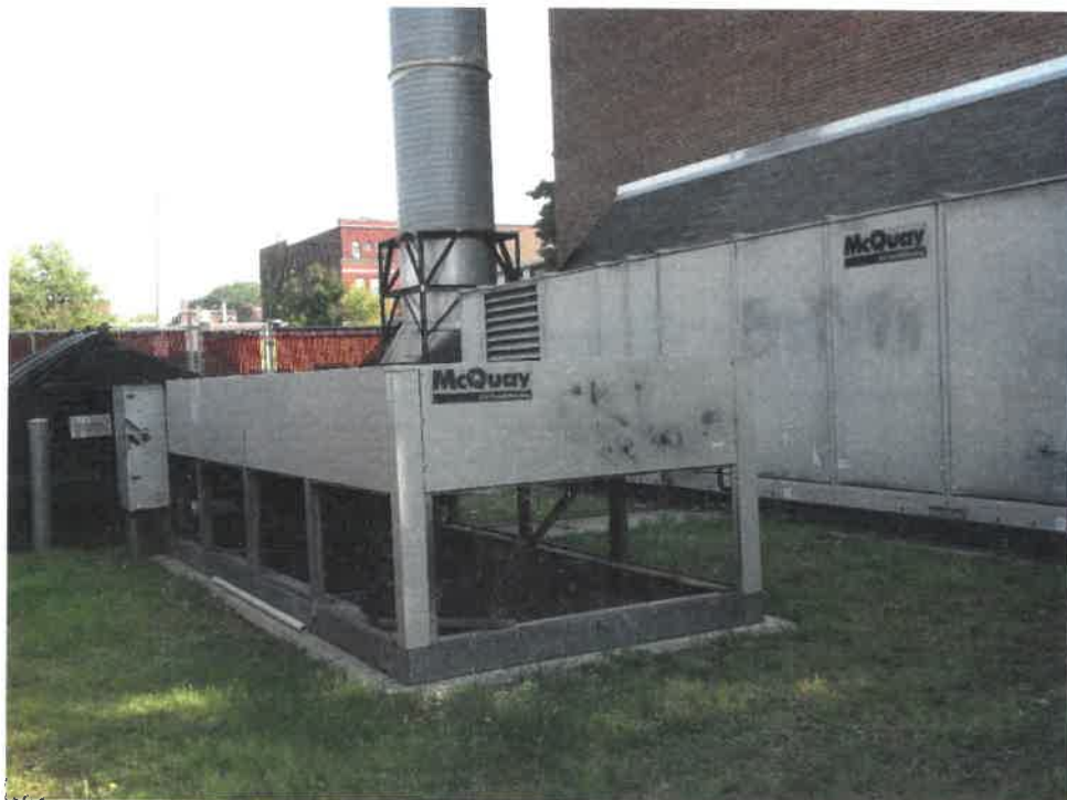
Figure 5 - existing HVAC equipment
