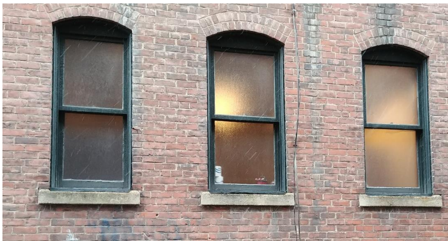
Above: A photograph submitted by the applicant depicting windows proposed to be replaced on the south façade of the Colonial Theatre building.
