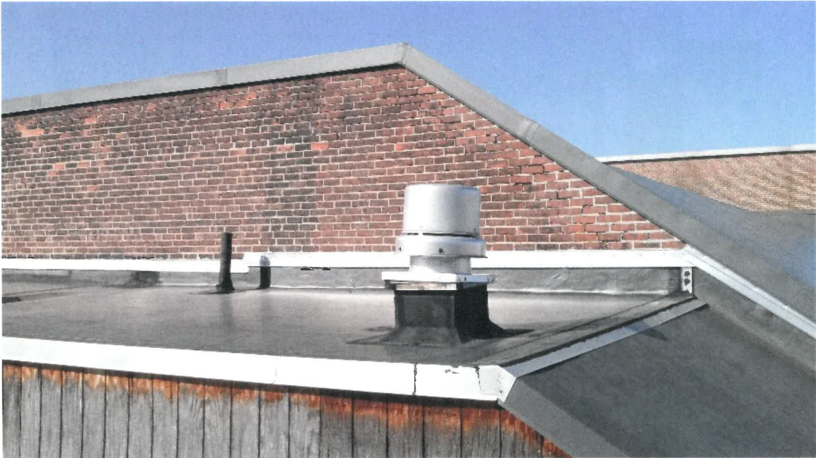
Figure 6 - example of brickwork requiring repointing
