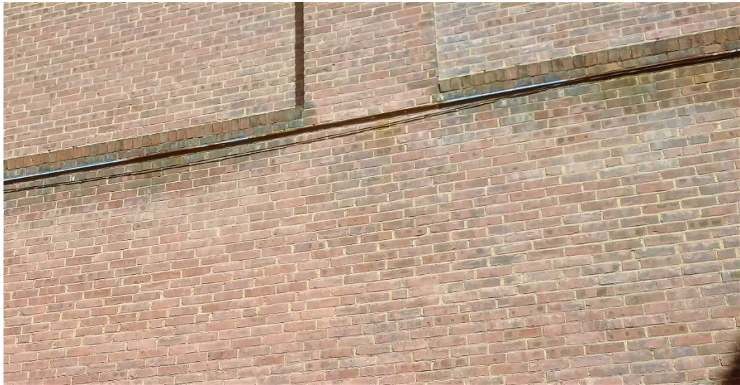
Attachment # 2 - Brick Staining South Walls
