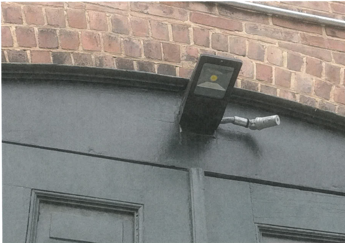
Figure 18 – Exterior lighting at exit doors
