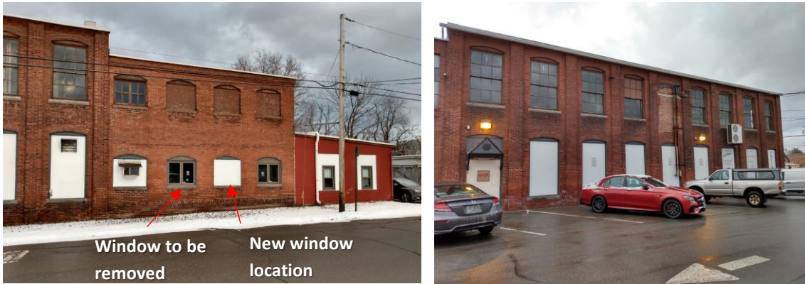
Figure 4 (Left): The current and proposed locations of the window to be relocated. Figure 5 (Right): Some of the windows on the first floor to be uncovered and repaired on the east façade.
