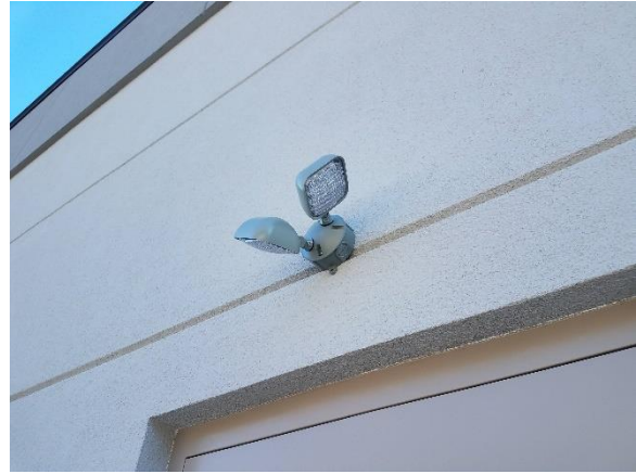
Figure 1. Photo taken on 2/14/20 of a light fixture installed above an egress door on the west facade of the Subaru building addition.
