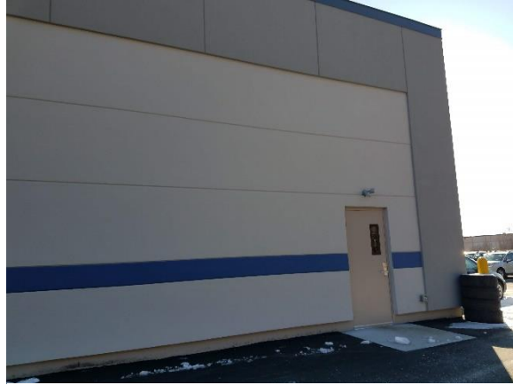
Figure 5. Photo taken 2/14/20 to show a portion of the west facade of the Subaru building addition, where a second egress door was installed.
