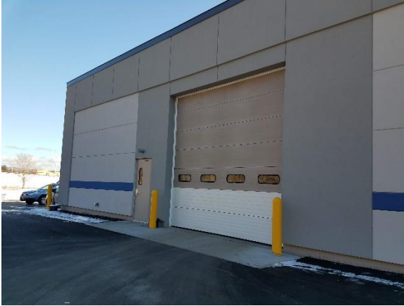
Figure 4. Photo taken 2/14/20 to show a portion of the west facade of the Subaru building addition.
