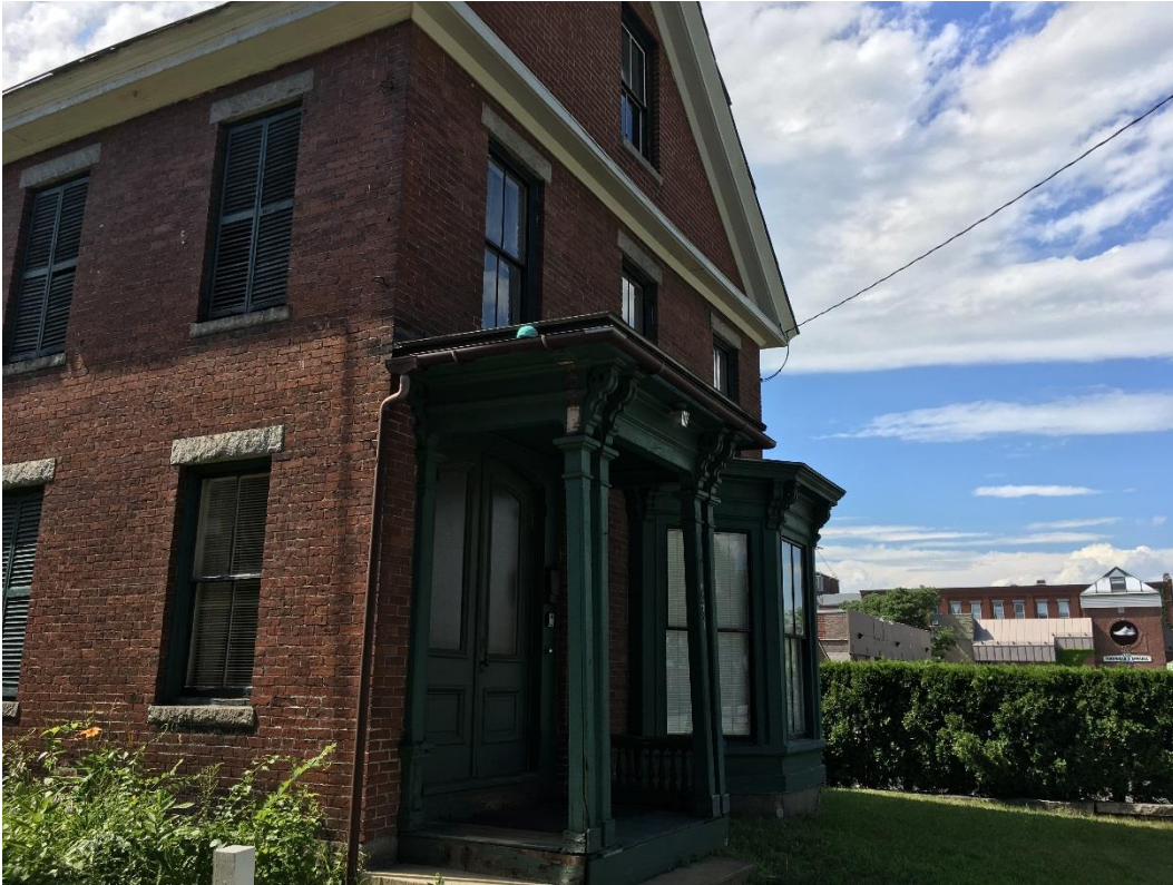
Image of front entry showing woodwork to be repaired and repainted and stairs to be reconstructed Shuttered windows to remain shuttered
