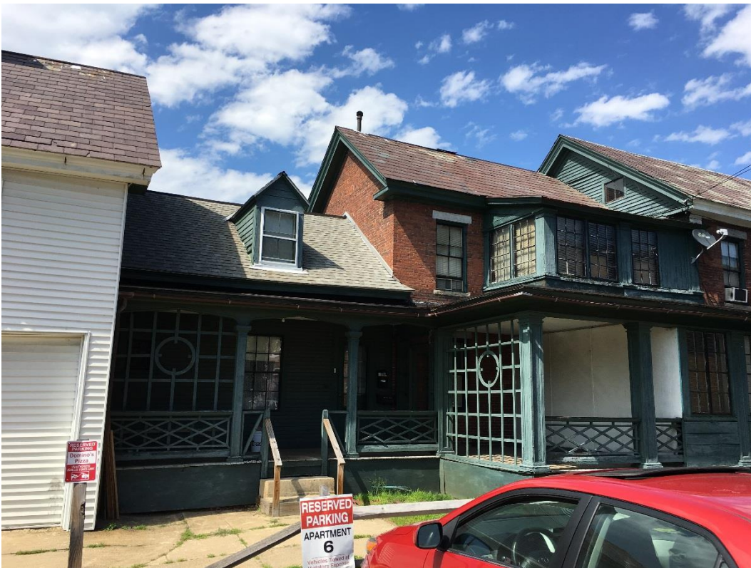
Image of woodwork to be repaired and repainted at side entry and slate roofs to be repaired
