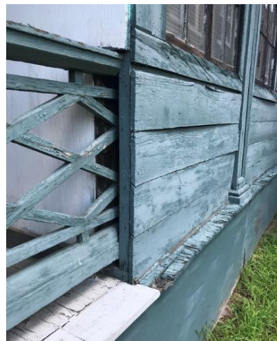
Figure 4. Image provided by the Applicant that shows where the porch railing is covered up by a wall.
