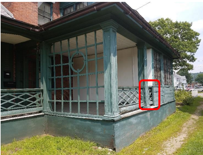
Figure 3. Image of the porch on the south side of the building that shows where the original porch railing was covered up by a wall (area circled in red). Photo taken by City staff in August 2018.
