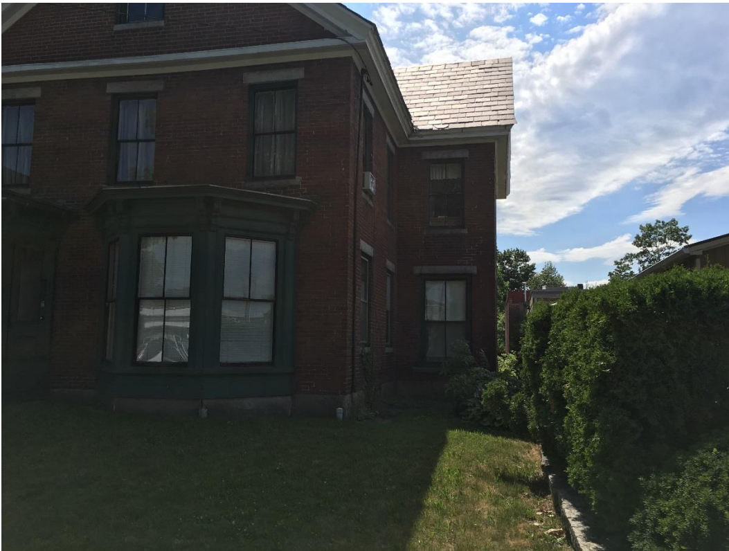
Image of windows to be replaced with woodwork to be repaired and repainted. Also shown is the typical state of the brick that will require repointing.
