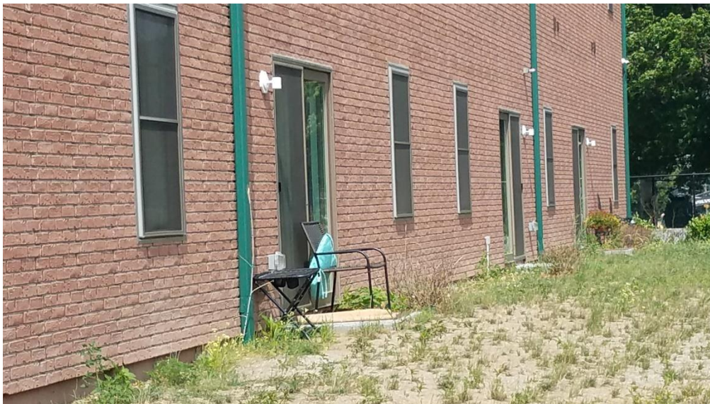
Figure 5. Photo showing light fixtures installed on the south facade of the building. Photo taken July 8, 2020.
