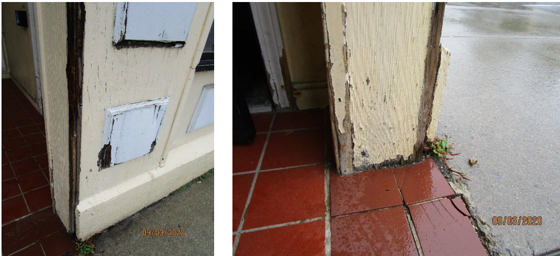
Figure 3. Photos submitted by the Applicant showing deteriorated portions of the existing wooden storefront trim. Photos taken September 3, 2020.
