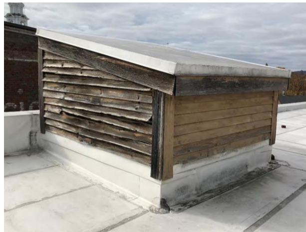
Figure 2. A photo submitted by the applicant showing the existing siding on the elevator penthouse.
