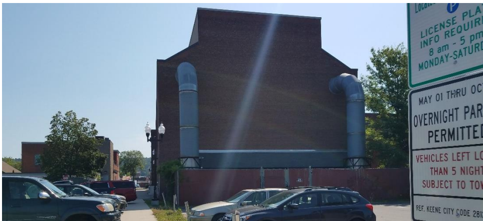
Figure 4. A photo of the exposed ductwork on the rear of the Colonial Theatre building. Photo taken August 6, 2019.
