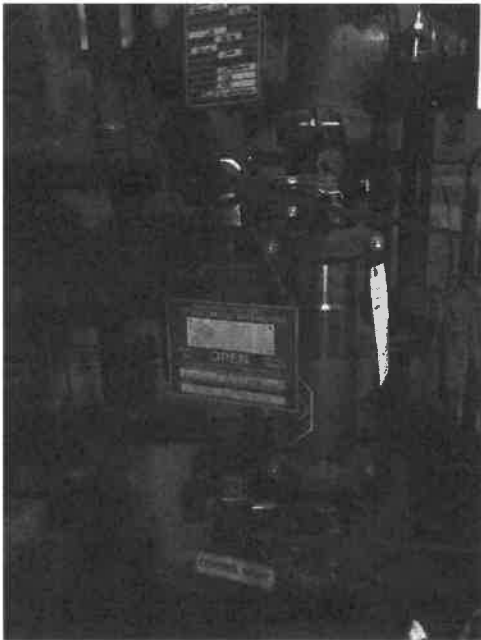
Sprinkler System Riser
