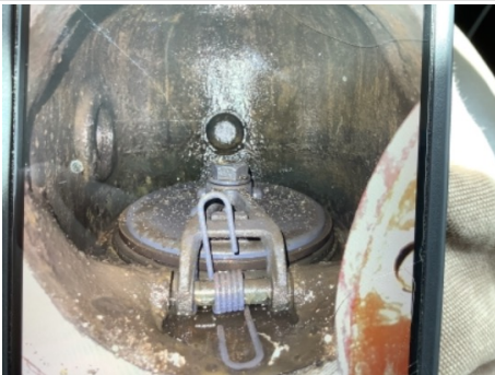
South Riser 6" Alarm Valve Internal
