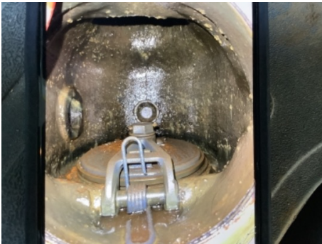
West Riser 6" Alarm Valve Internal
