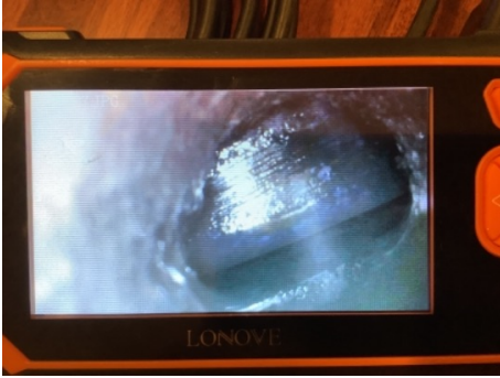
North Riser 6" Alarm Valve Internal
