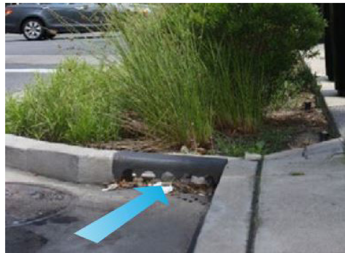
A grated inlet prevents large floatable trash
