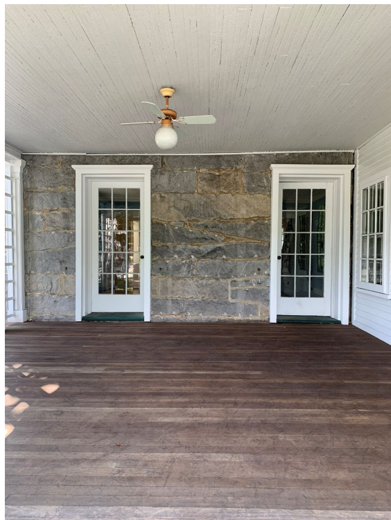
Figure 3: Porch doors to be replaced
