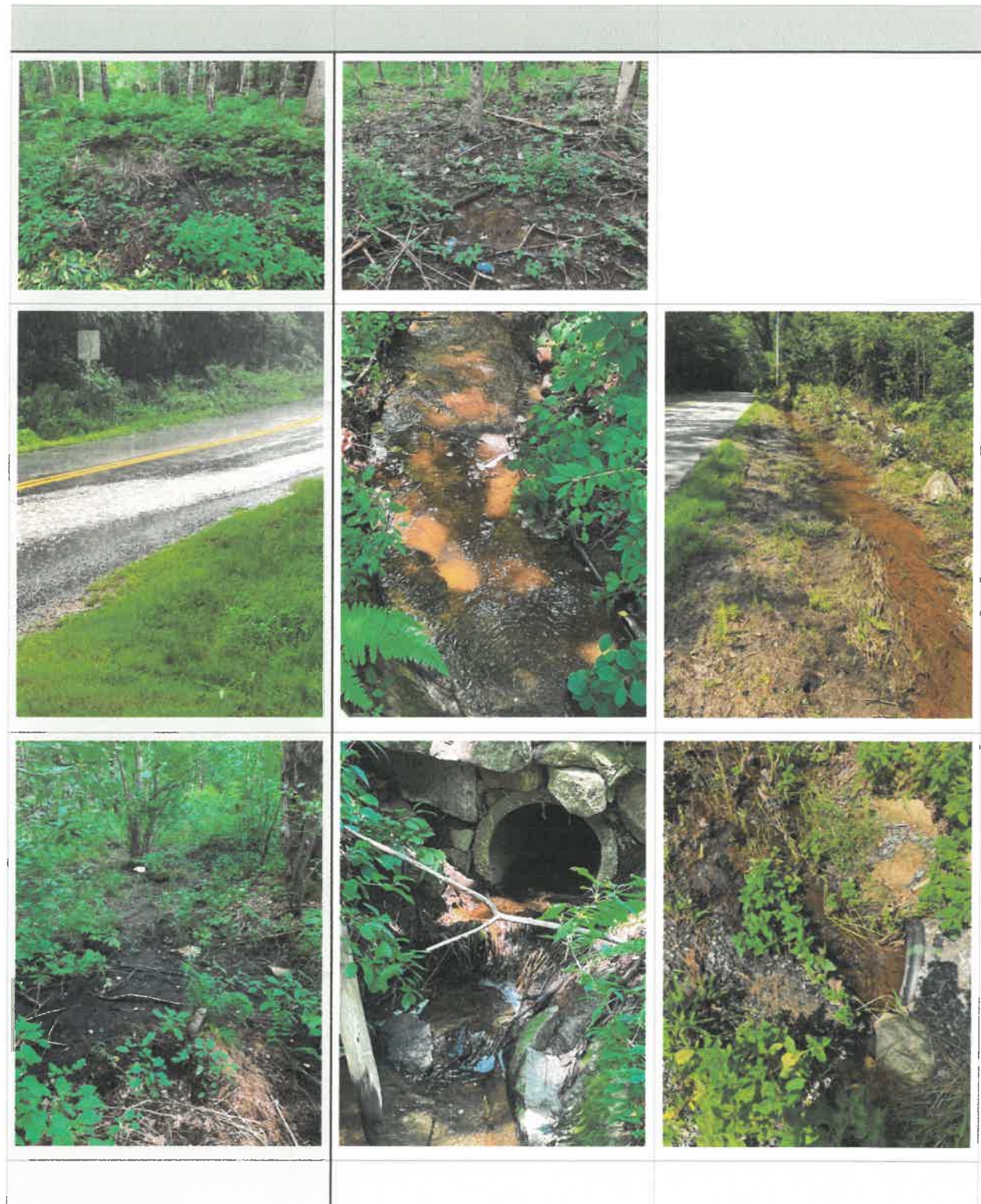
Various photos showing rain water flowing into the Habitat property on Old Walpole Rd. creating very wet soil conditions.
