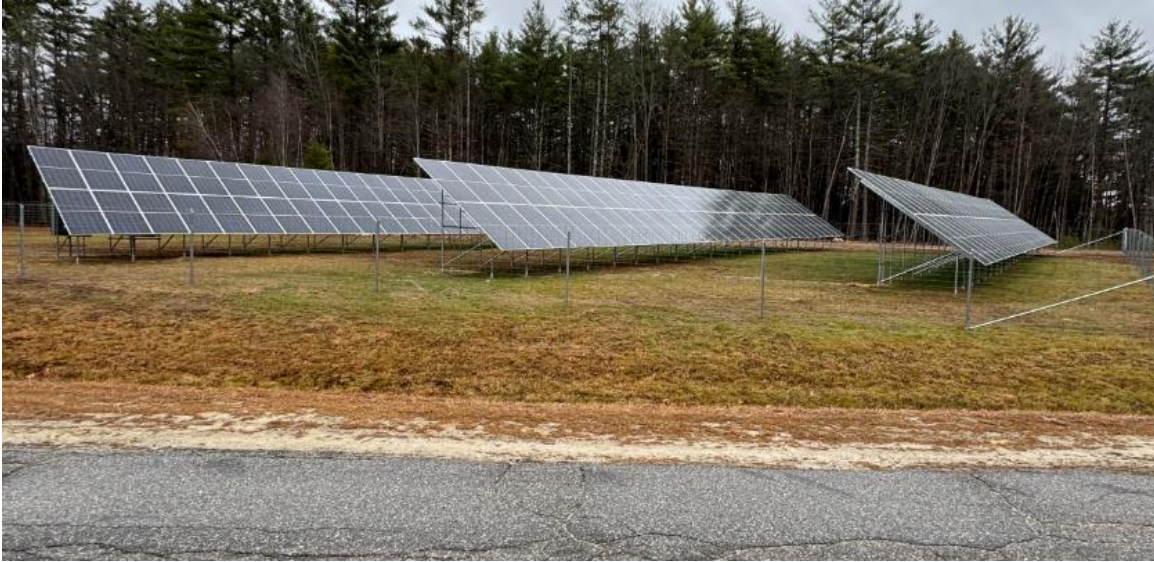
Example Photo of Solar Panel front view with APA racking system
