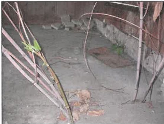
Structural damage to residential home/basement
