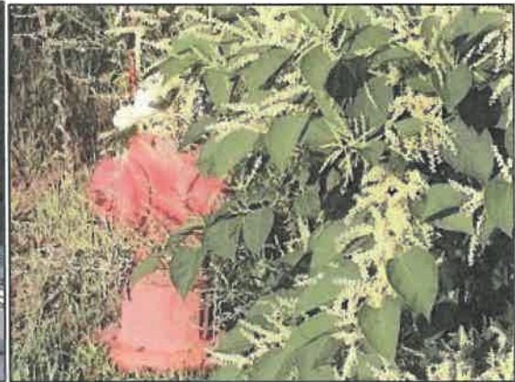
Obstruction of fire hydrant
