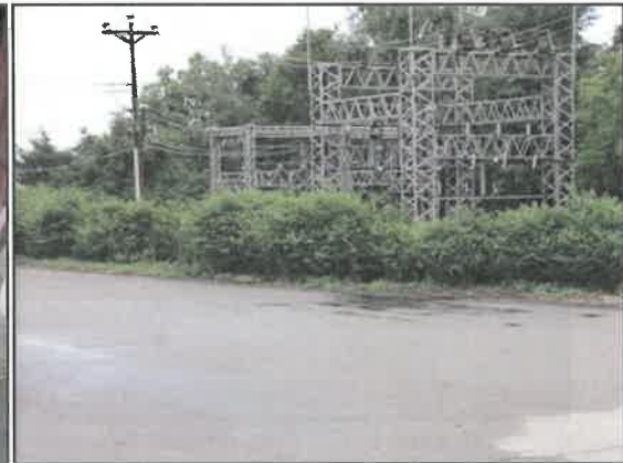
Power grid sub-station impacts
