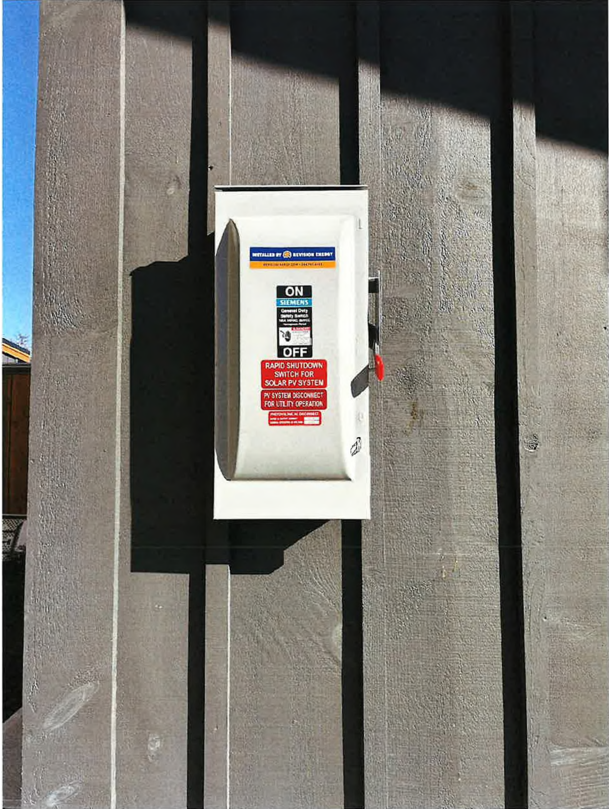
100A exterior disconnect up close
