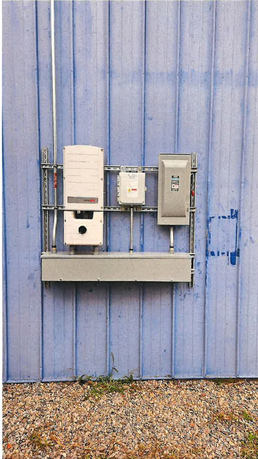
17.3kW Inverter w/ 100A exterior disconnect (if inverter had to be outside)
